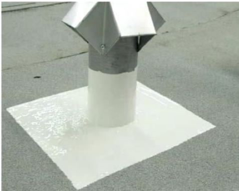
Fig. 7b: Coat over Ply-Flash Compound with compatible coating after allowing compound to cure/weather 30 days.
