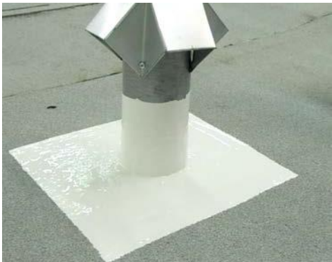
Fig. 7b: Coat over Ply-Flash Compound with compatible coating after allowing compound to cure/weather 30 days.
